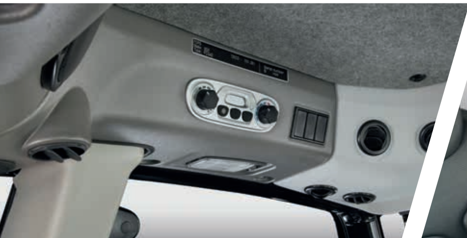
> Air conditioning controls.
